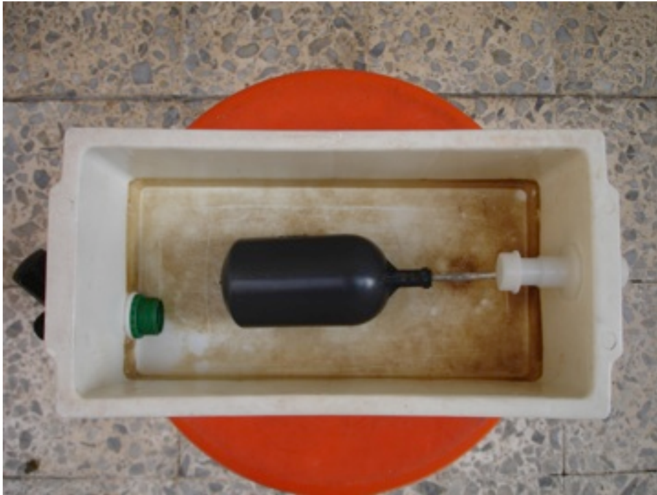
Photo 6 – Valve fixed inside box
