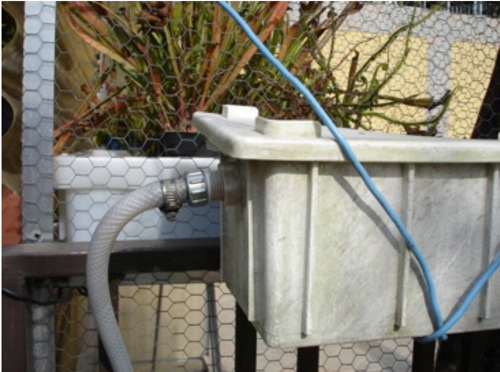
Photo 18 – Hose connected directly to the valve
