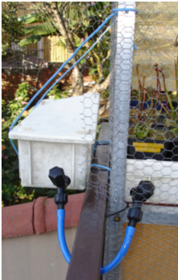
Photo 13-a - Box and tray connected
